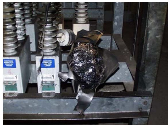
Figure 2 – Example of physical damage caused by harmonic resonance
